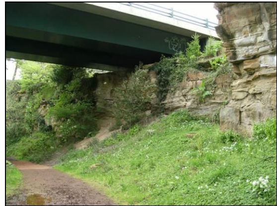
Photo ELC_17 P7: Cliff section continues along the east bank of the River Esk and has been used as a foundation for the A68 which crosses the river at this point. © BGS, NERC.
