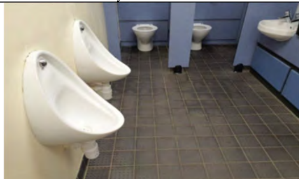
Photo 17: Concealed bitumen-based flooring adhesive (Chrysotile): Sample No: S0068: Room No: B01/FG/R031: Boys Toilets
