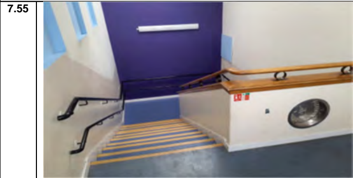
Photo 55: Concealed asbestos containing floor tile adhesive (Chrysotile): Sample No: S008: Room No: B01/FG/R022A: Circulation Area / Staircase Mid Landing
