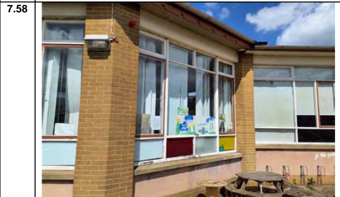
Photo 58: Asbestos containing mastic to windows frame sides (Chrysotile): Sample No: JP000701: External Elevation No: EXT001
