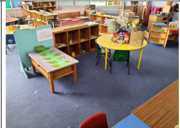
Photo 9: Concealed bitumen-based flooring adhesive (Chrysotile): Sample No: S0049: Room No: B01/FG/R008: Classroom
