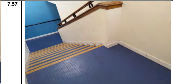
Photo 57: Concealed asbestos containing floor tile adhesive (Chrysotile): Sample No: S008: Room No: B01/F1/R022B: Circulation Area / Staircase Mid Landing
