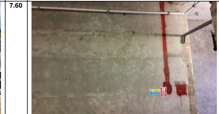
Photo 60: Sealed asbestos thermal insulation debris to Wall 9 (Amosite & Chrysotile): Sample No: IOM30A: Room No: B01/FB/R001: Former Boiler House
