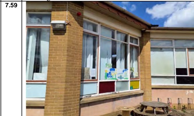
Photo 59: Asbestos containing mastic to windows frame sides (Chrysotile): Sample No: JP000702: External Elevation No: EXT001
