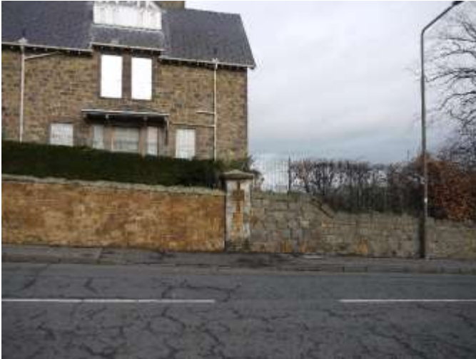
Western boundary to Aberlady Road adjacent to south-west pavilion, illustrating variety of stones, bonding and coping styles
