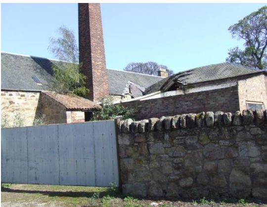
Figure 89 Pinkiehill Farm has deteriorated since becoming vacant
