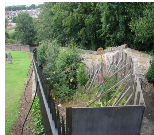
Figure 101 The walls at the graveyard on the edge of the brae have been hoarded off for many years and require repair
