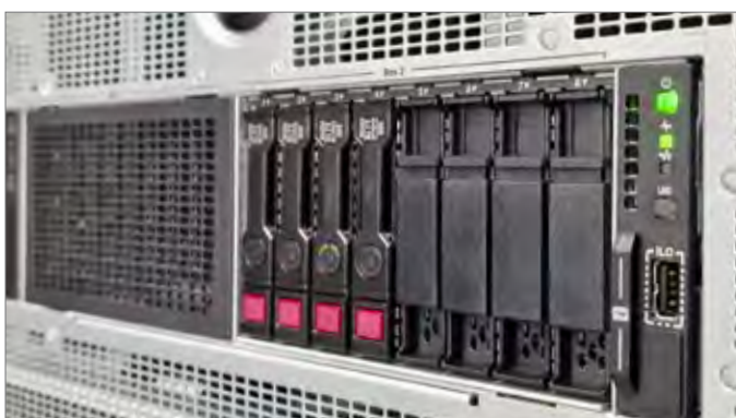
Apollo Server (housing GPU Processors)
