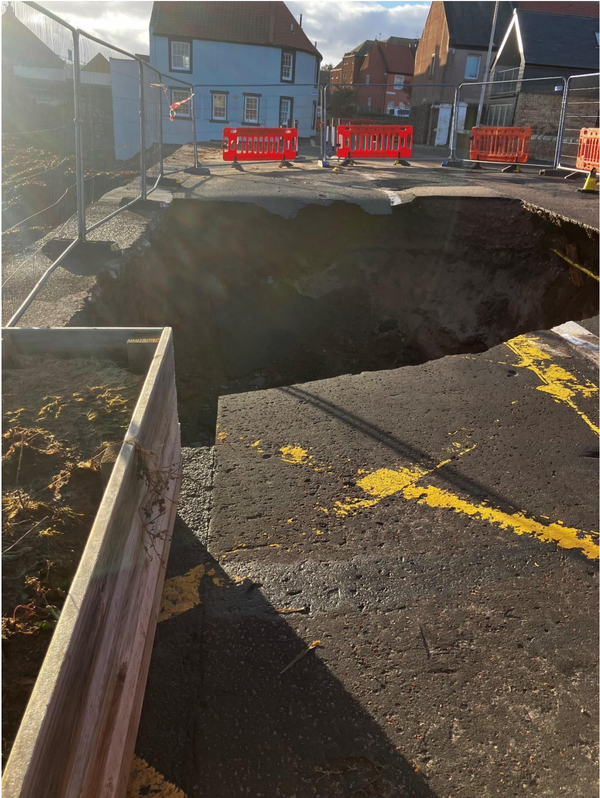
Sinkhole at Lamer Street, Dunbar
