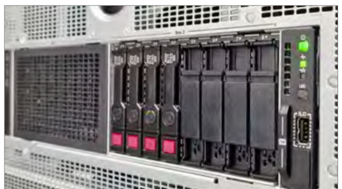
Apollo Server (housing GPU Processors)
