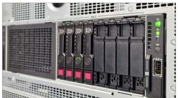
Apollo Server (housing GPU Processors)
